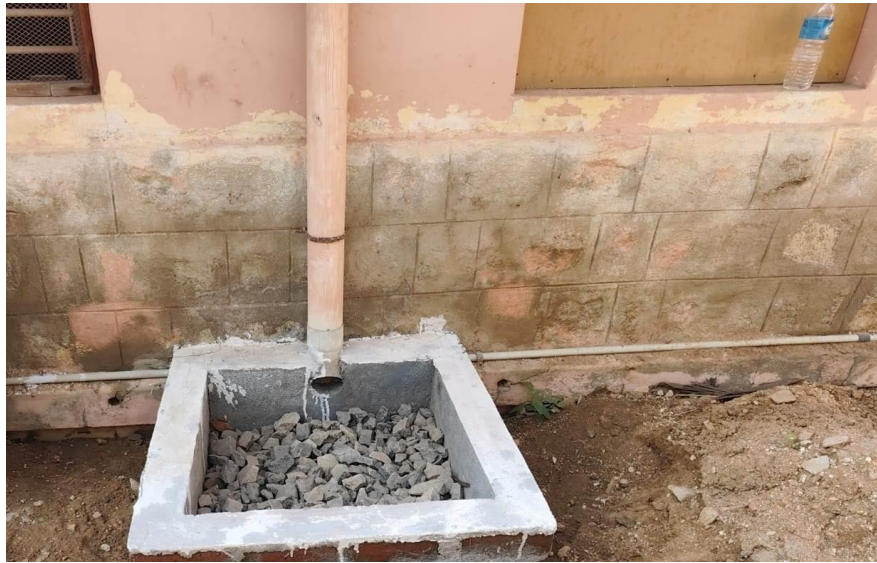
Rain Water Harvesting Pits inside the campus
