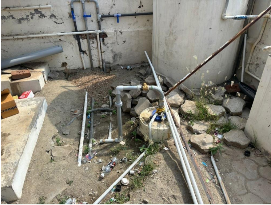
Recharge Bore well inside the campus
