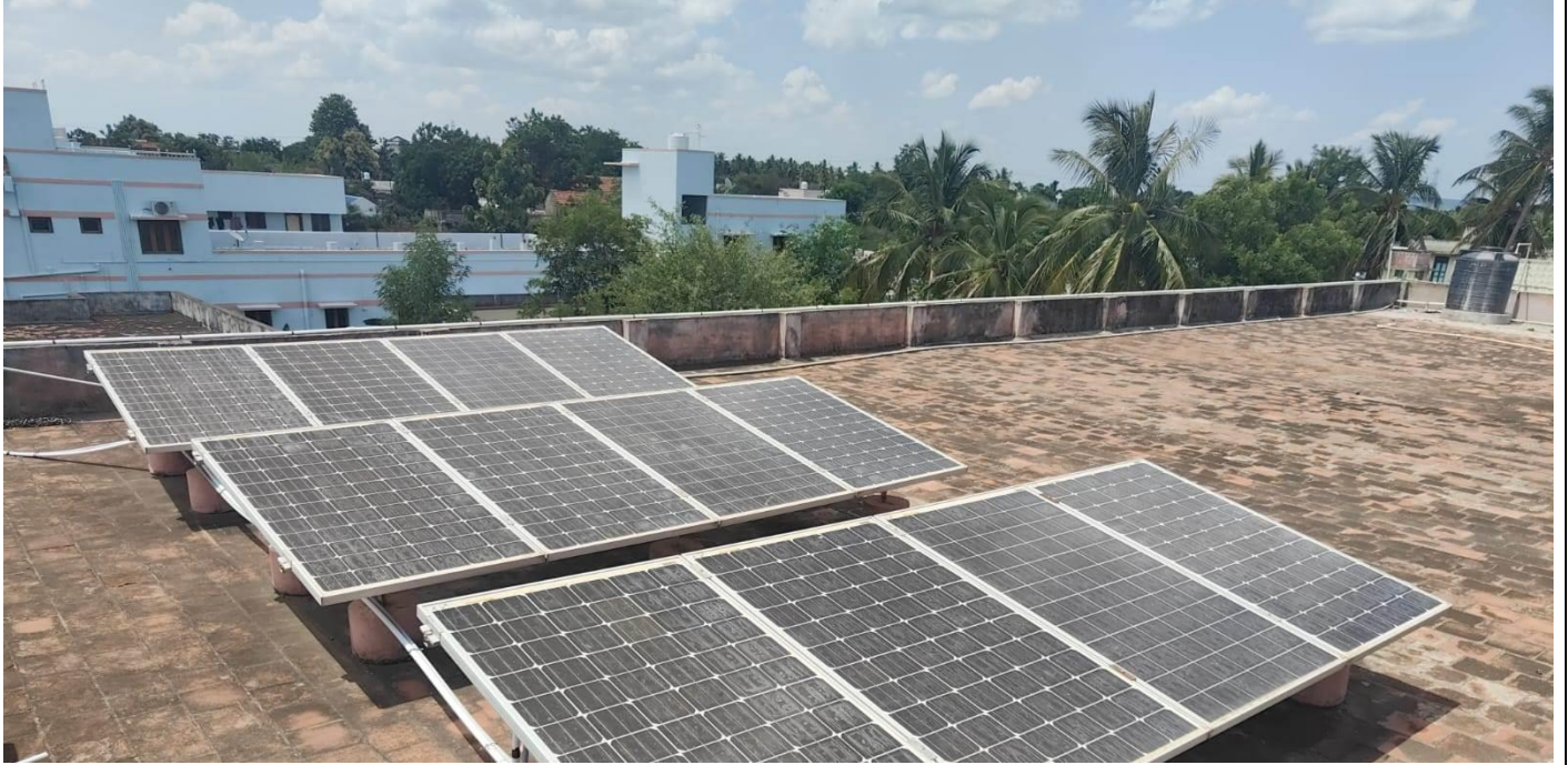
Solar panels in all around the campus
