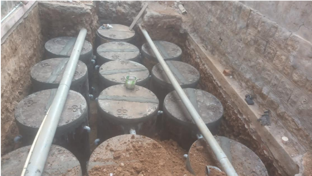
Bio water Treatment Process inside the campus
