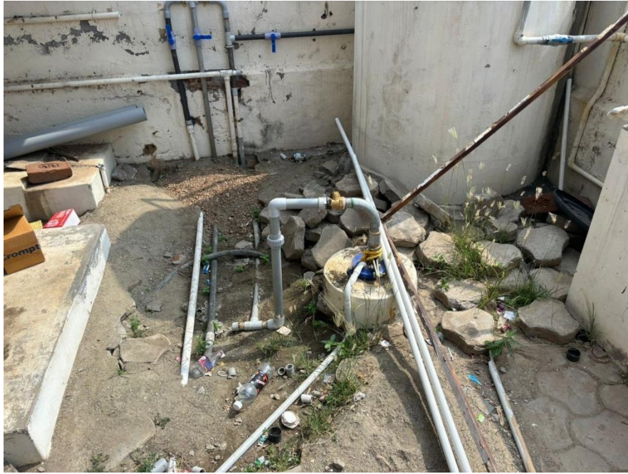
Recharge Bore well inside the campus
